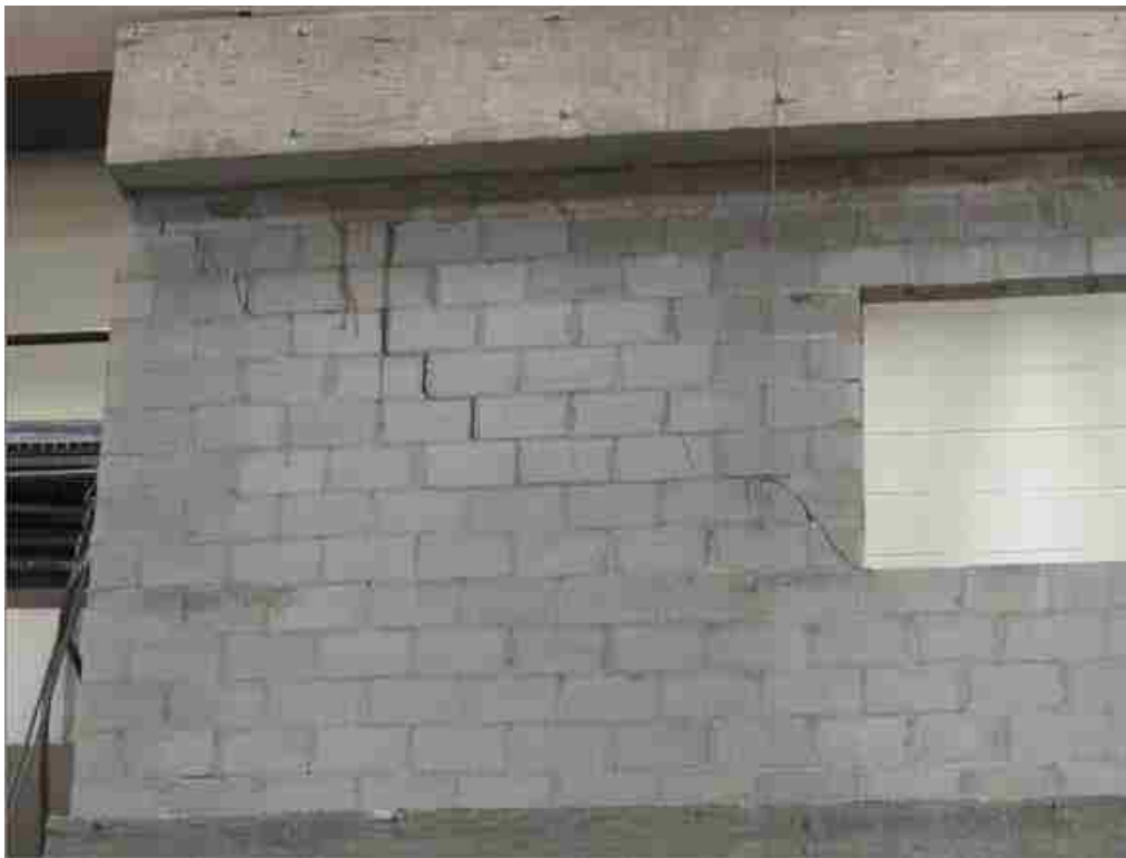
Figure 4-6: Diagonal cracks stepping through mortar joints
